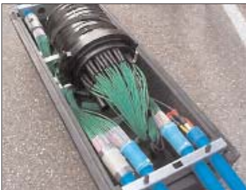
Blown cable FTTH application
