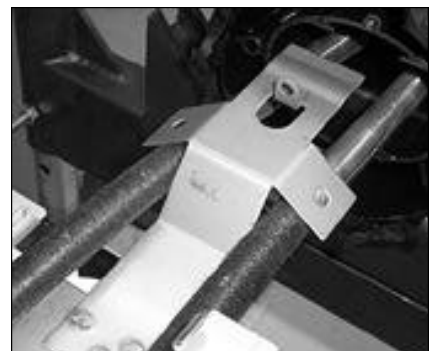
24. Place organiser in between the cables and fit to the base, secure using the screws.
