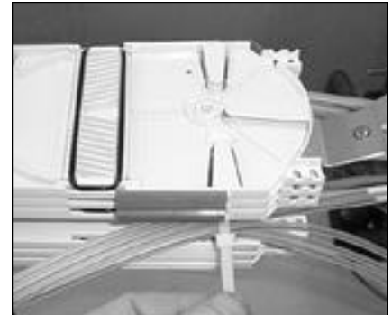
21. Loop a cable tie over all of the units near the base. Tighten until the units on both sides are in line with the trays.
